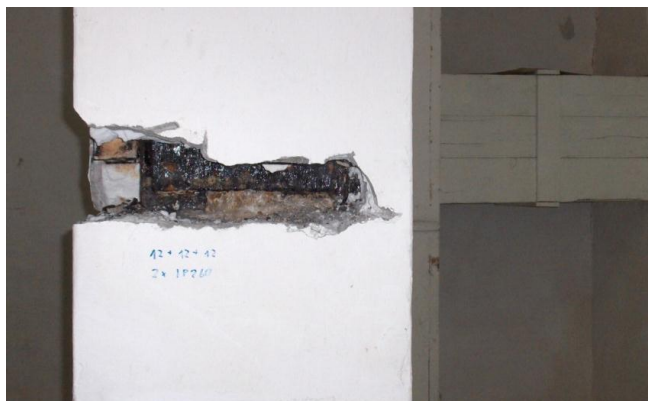
Fig. 3. "In-situ" inspection hole of the steel supporting structure of the column. Visible degree of column corrosion.
