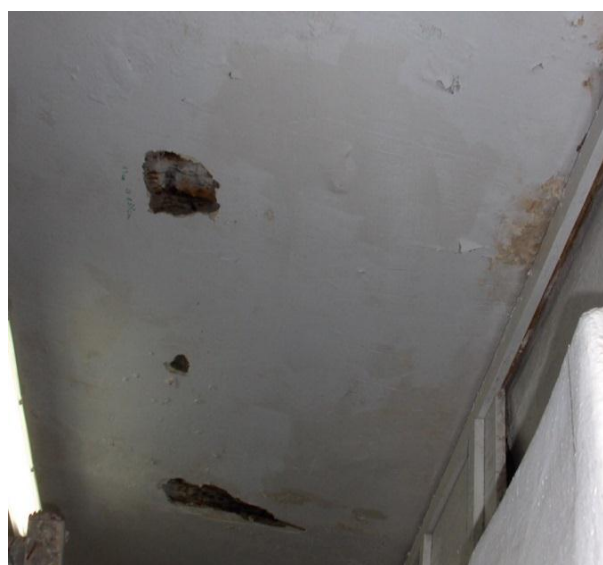
Fig. 2. “In-situ” inspection hole of Klein ceiling beams in a cold store in Warsaw
