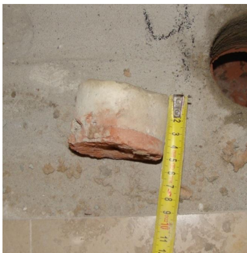
Fig. 1. Measurement of the thickness of the concrete slab-overlayer of the Ackerman block ceiling
