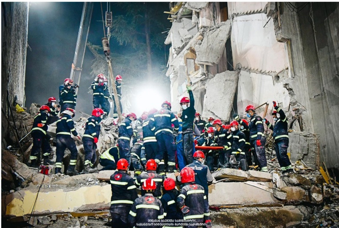
The illegal construction works lead to the eventual collapse of a section of the residential building causing the death of 9 people, including 3 minors.
