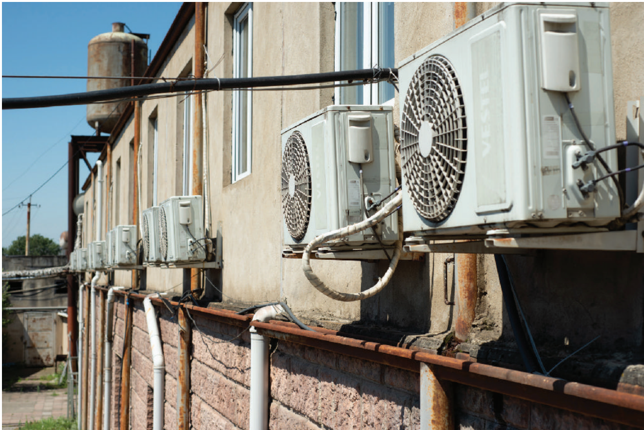
In Kutex, only the administration's offices are air-conditioned, despite the oppressive summer heat on the factory floor. Photo: Tamuna Chkareuli/OC Media.
