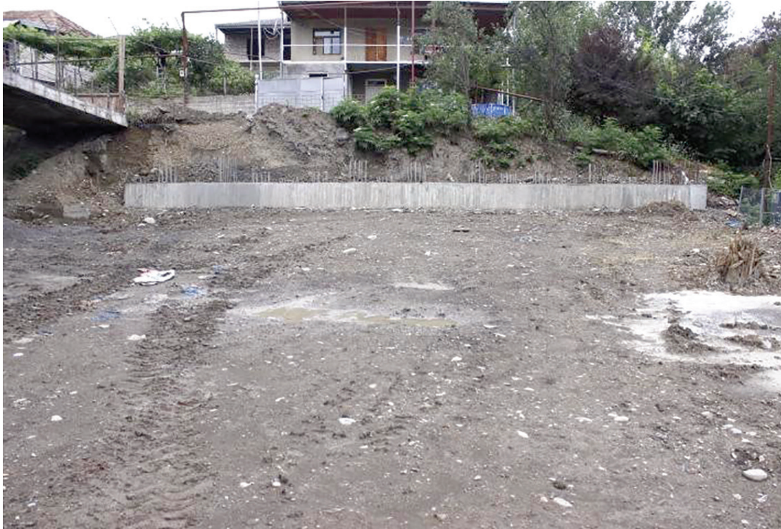
Fig. 4. The area of the hollow before the land is removed. Retaining wall in the background
