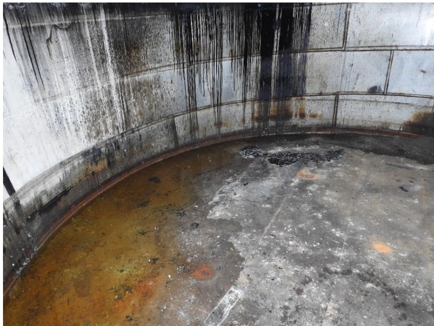
Fig.1. The bottom of the first tank
