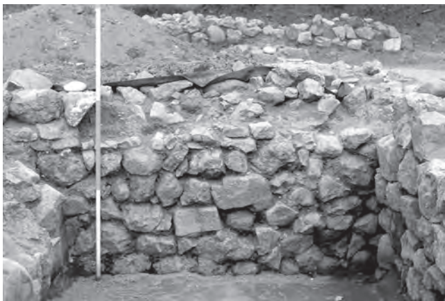
Fig. 8. Gonio (Sector NO 01, Square 97). The face of wall W2 (view from the west). Visible ventilation hole secondarily blinded with an additional stone. © A. Trzop-Szczypiorska
