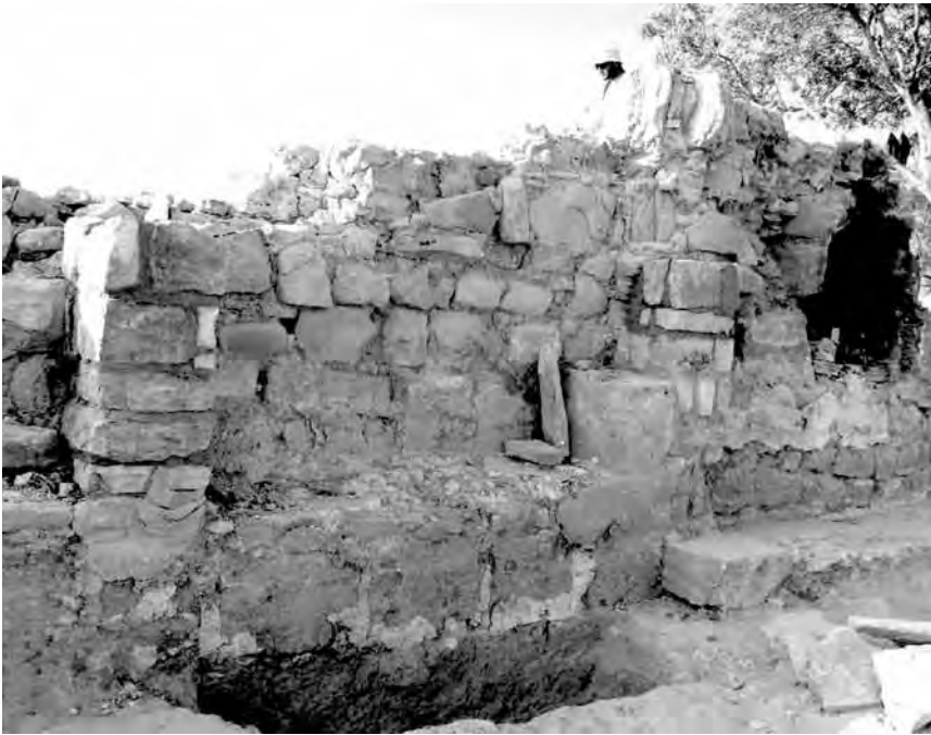
The partial restoration of the Northern wall and the pilasters of Alaminos church
